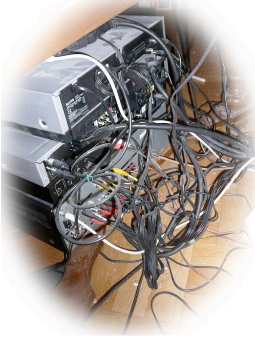
Figure 4. The reality behind a “normal” installation of the system. Additional wiring was required apart from what was shown in figure 3. (Photo and wiring by the author)
